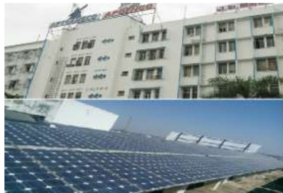
Fig 2.1 Arrangement of PV arrays at Vidyut Soudha
